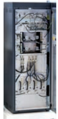
Cassidian's new TB3S TETRA base station.
